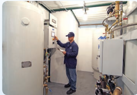
AS-J250-HPCR Containerized High Purity Packaged PSA Oxygen Plant for NATO Forces — Afghanistan
